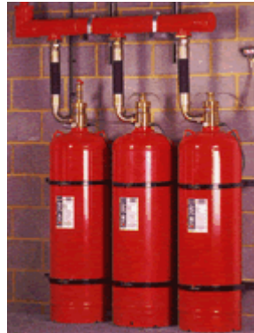
Figure 7 – Gaseous agent cylinders
